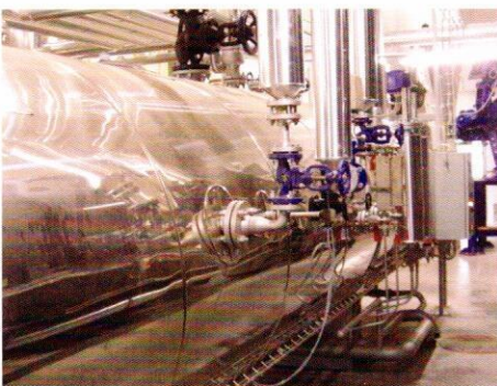
Waste Heat Boiler
