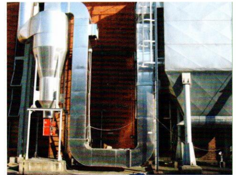
Cyclone with Bag House Filtration
